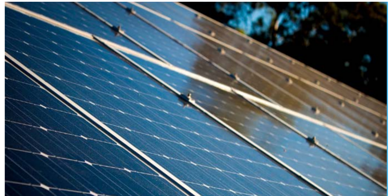
Image 20: Sensitive installed photo voltaics
